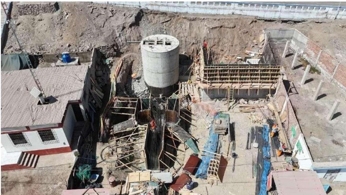
Aerial view of progress on the CBD-03 Drainage Pumping Chamber, the most important chamber, as it will pump wastewater collected from all of Chala to the PTAR.
