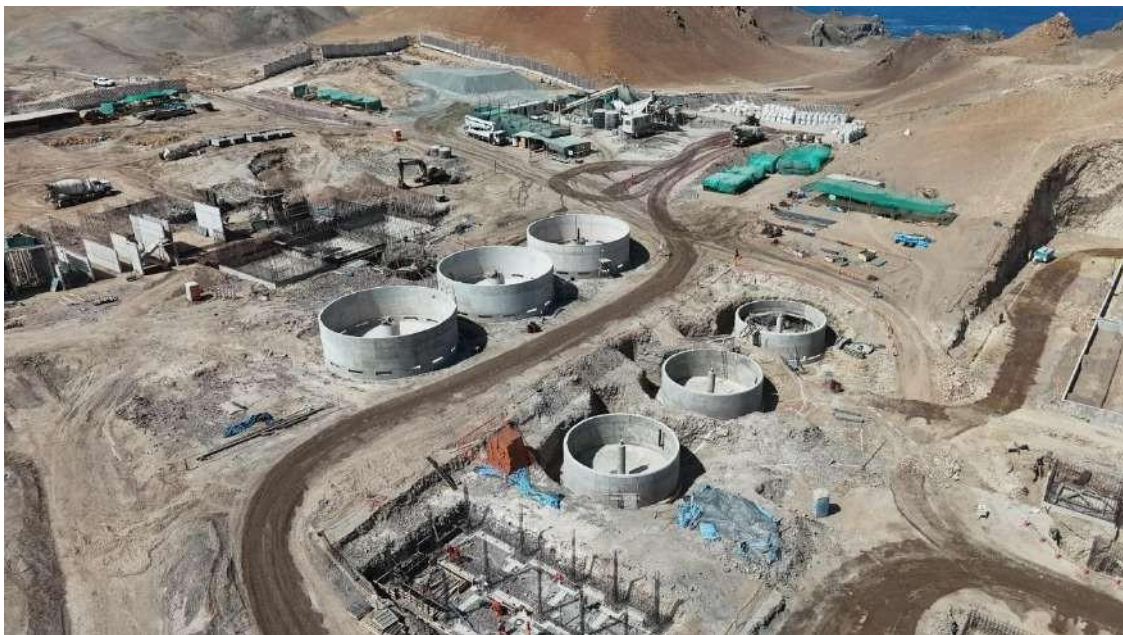
Aerial view of the PTAR – Chala, with its main components under construction, percentage of progress in civil works at 53%
